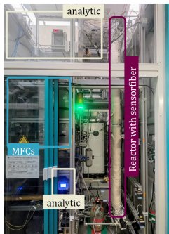
Reactor for the catalytic CO 2 methanation
